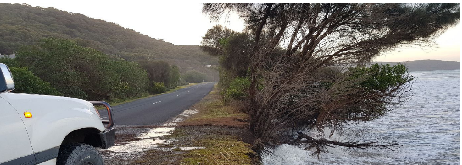
Wave erosion undermining road – Walkerville
