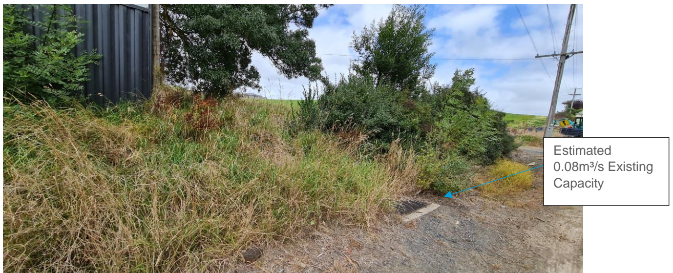
Figure 27. Existing Grated discharge at NE Corner
