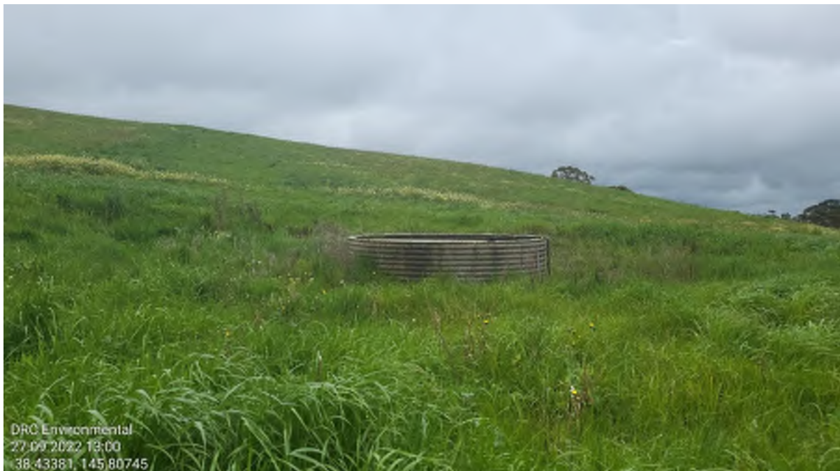
Plate 4: Concrete Water Tank present towards the north side, sealed off on top with one pipe connected to the water tank that runs into the ground
